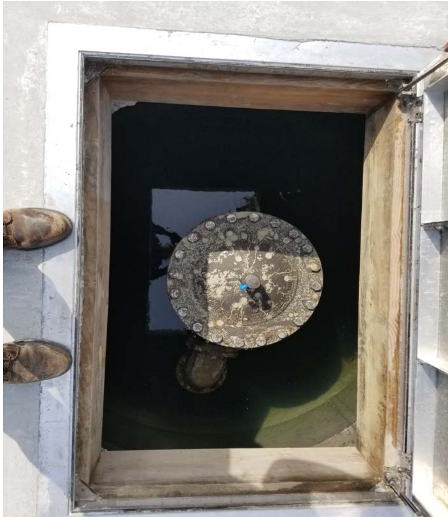
After installation, position of the pig injection port in comparison to pit hatch has improved dramatically.
