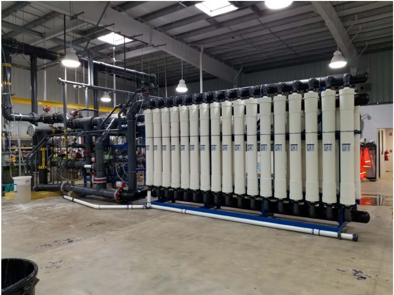
Fully Installed and functional Toray filter train.
