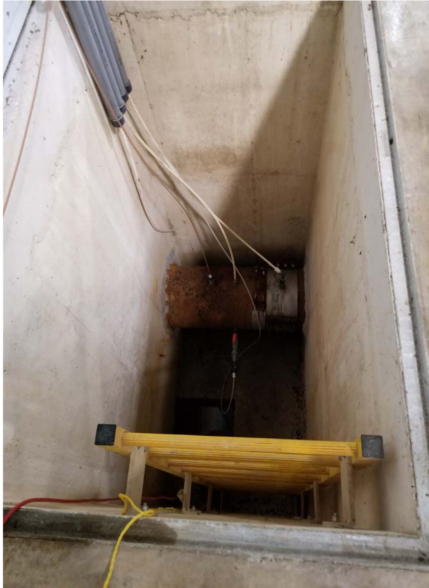
New Ammonium Sulfate feed point after the clearwell.
