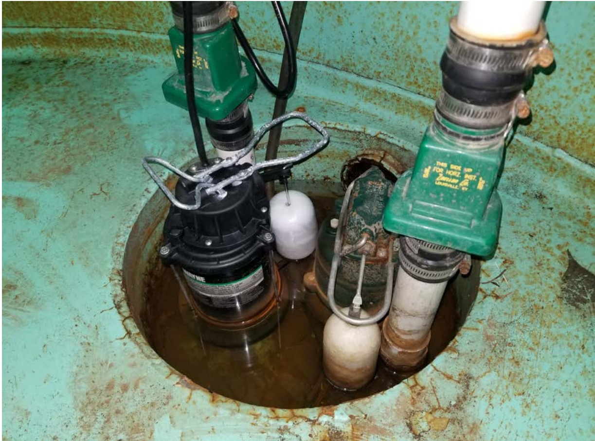
One of the sump pumps in the booster station failed. The check valve also failed allowing water to build up in the station. Cleared the check valve and replaced the sump.
