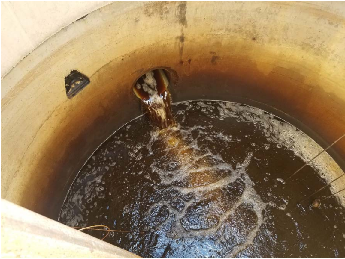
The backwash influent pump basin as we backwashed softener #2
