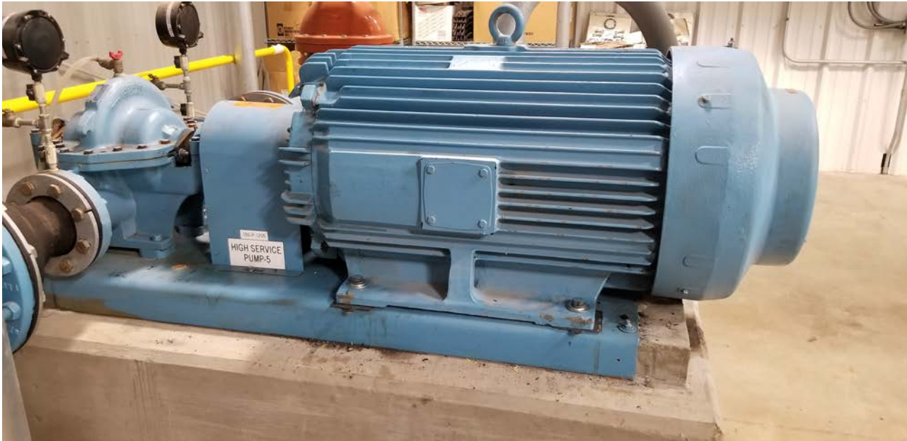
Hsp #5 rebuilt by Bodine Electric
