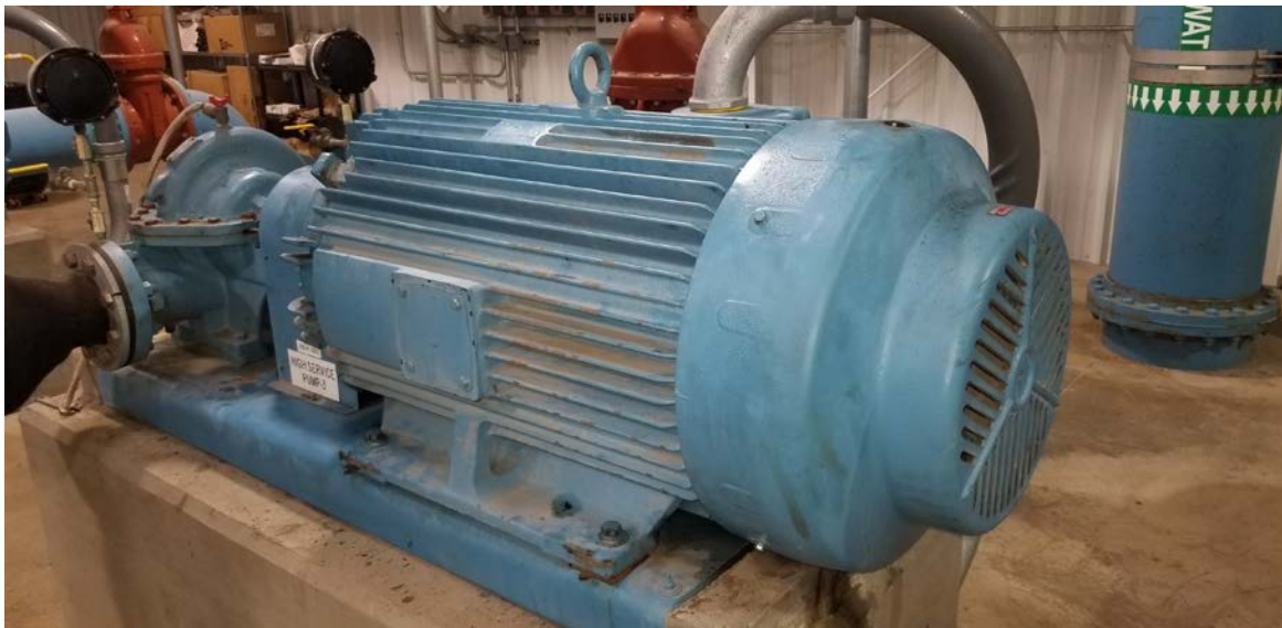
HSP #3 was rebuilt by Bodine electric
