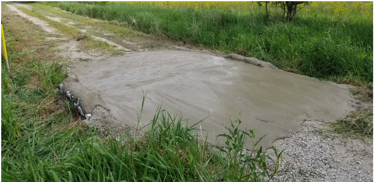
Washout in well that we repaired with left over well grout.
