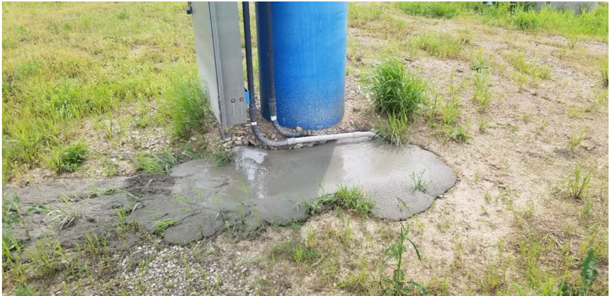
Grout in well #4 subsidence
