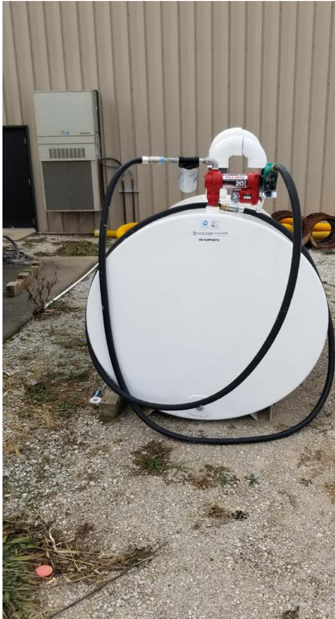
New diesel pumps installed
