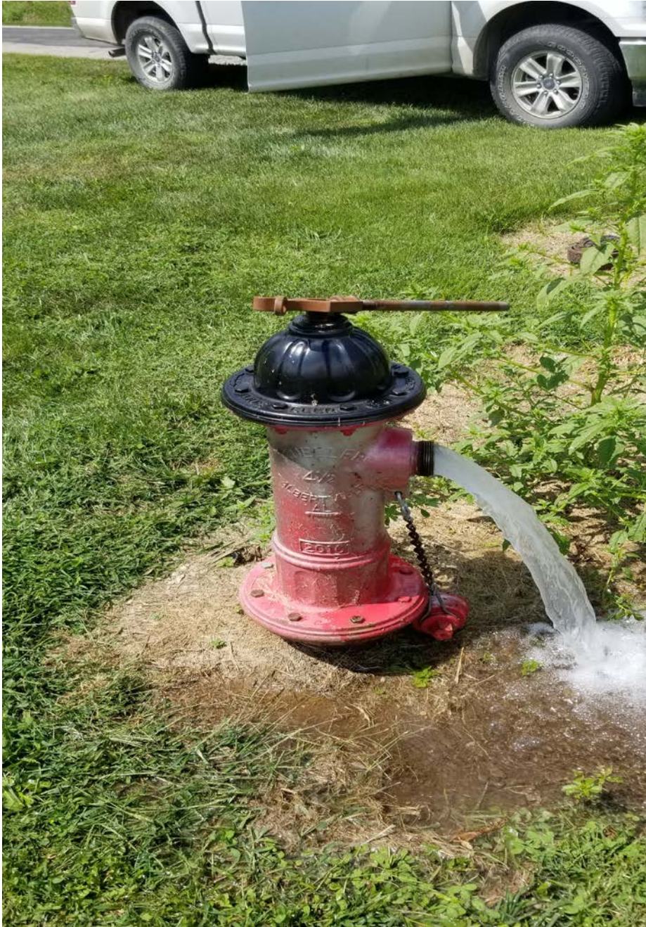
Preparing to draw a sample from a hydrant we had been flushing
