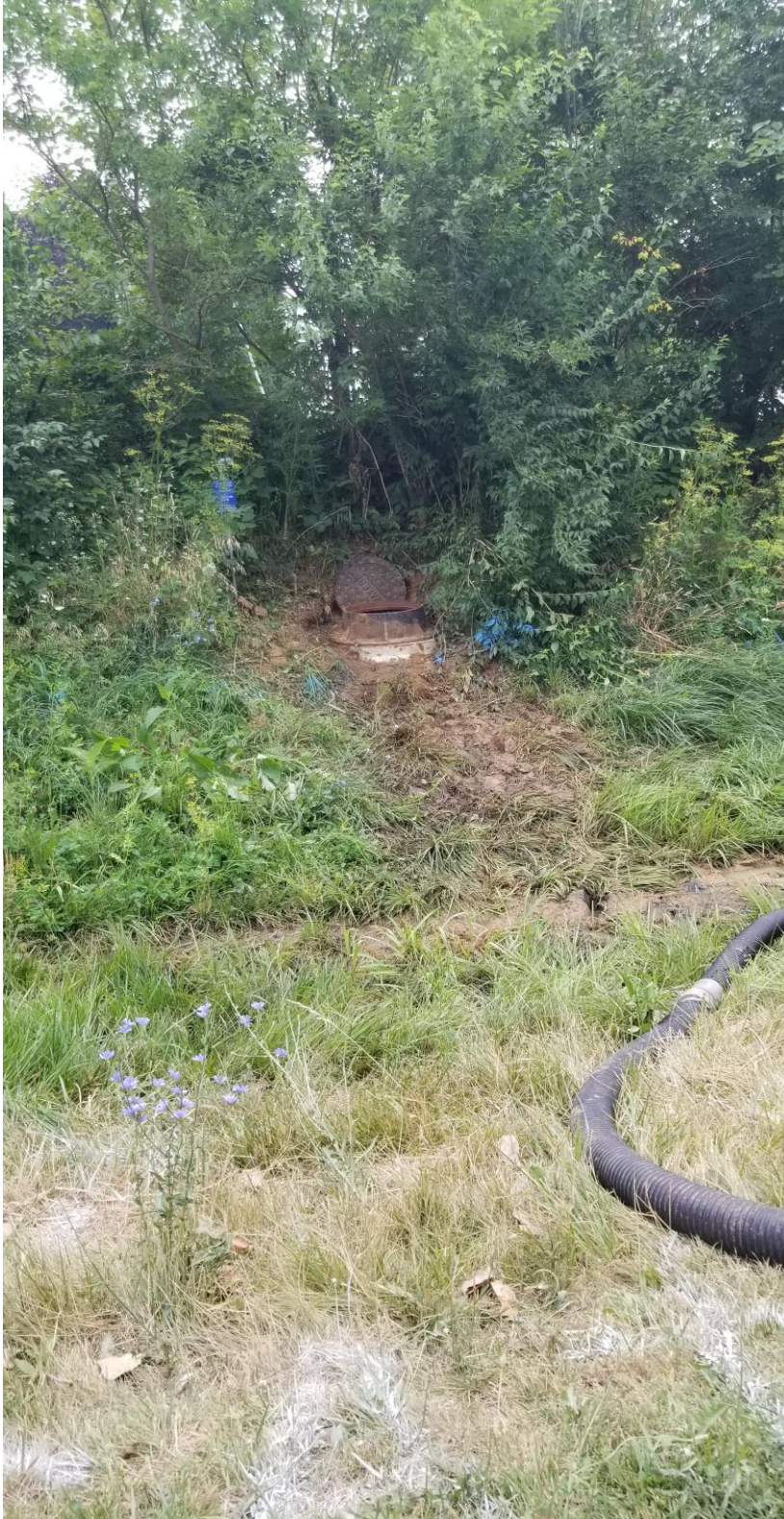
An air valve on Cardinal Hill Rd was leaking. We had Steve Ray Plumbing on site to cap the leak.
