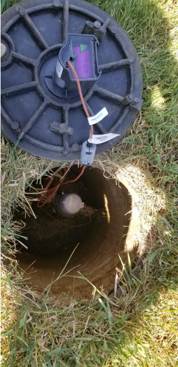
New cell transmitter installed on Mendenhall meter
