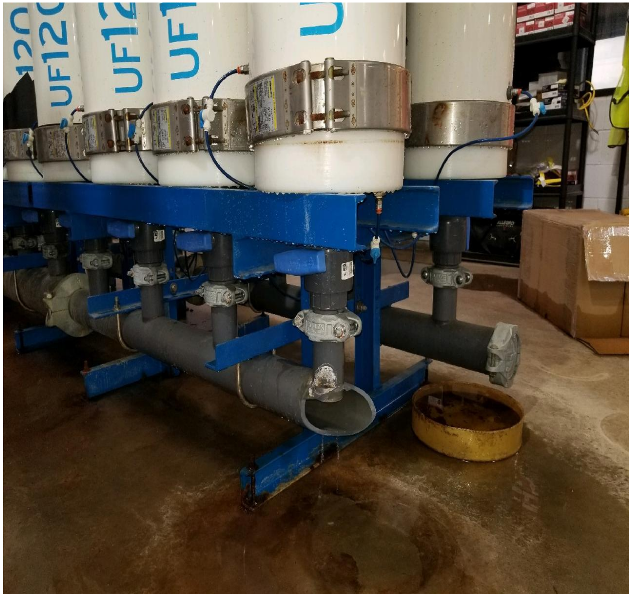
Filter train #3 was damaged when a filter comm loss occurred causing the train over pressurizer.
