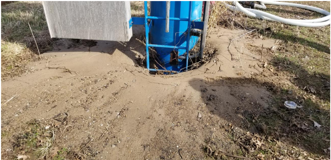
While cleaning well #3 Brotke broke ground causing a hole to form.
