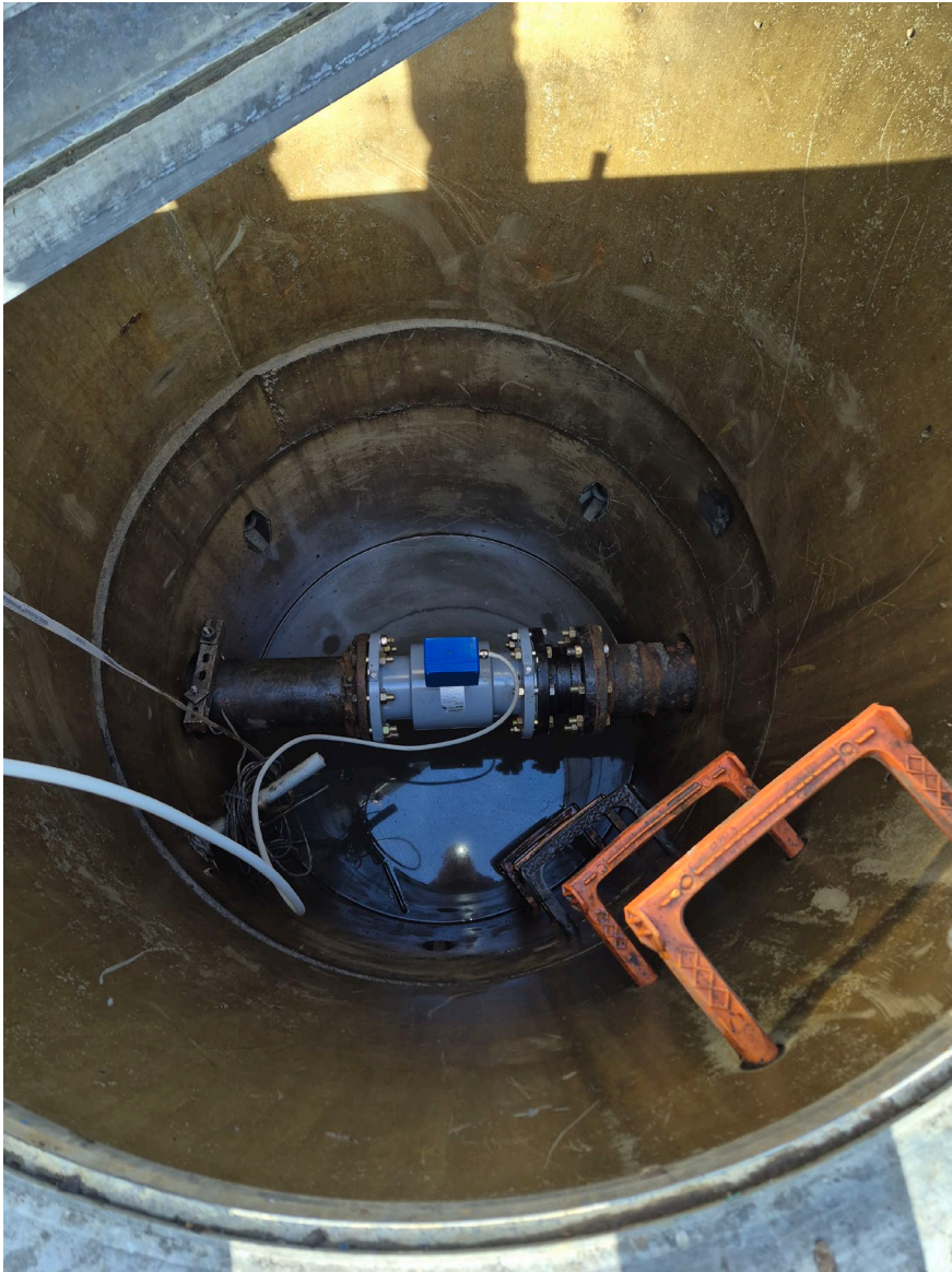
Well #10 new flow meter
