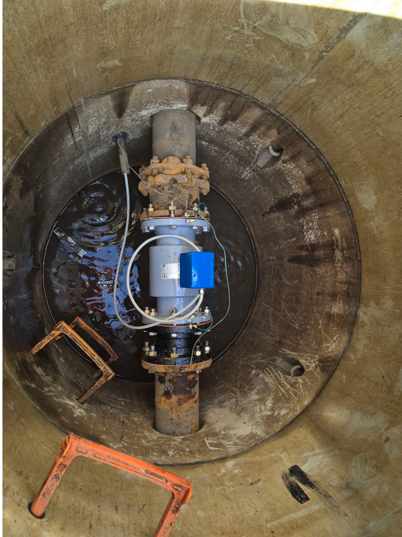
Well #8 new flow meter
