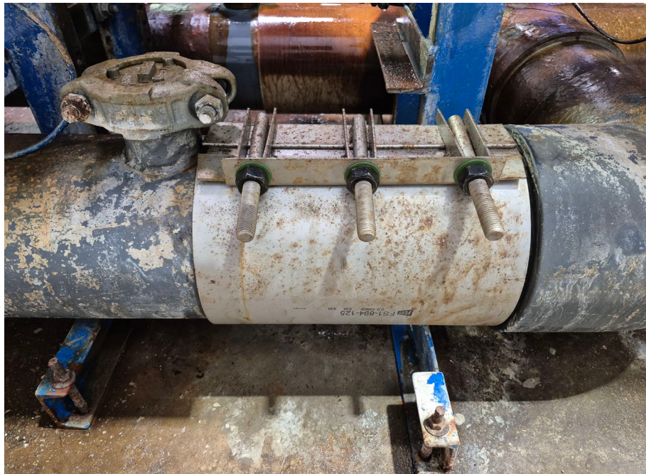
Train #3 leak and repair
